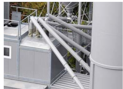
Siloanschlüsse Silo connections
